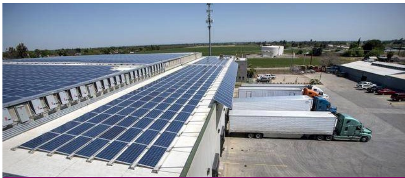
THE CALIFORNIA SUN BEATS DOWN ON A BRAND NEW SOLAR ARRAY ATOP PATTERSON CAOMPANIES' 210,000 SQUARE FOOT DISTRIBUTION FACILITY IN DINUBA, CALIF.
